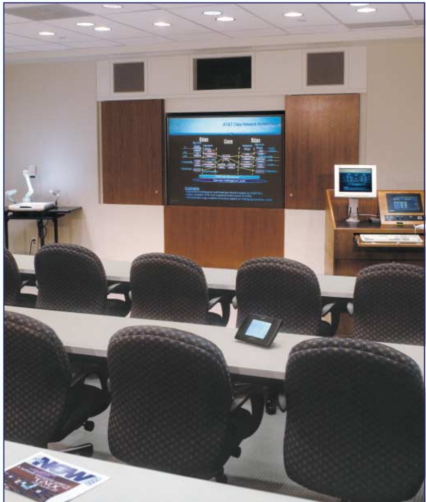
AT&T Network Operations Center, Bedminster, NJ. Installation by Vistacom, Inc. The project included five Retro/QA units, each with a 67" diagonal DiamondScreen. Photo courtesy of Vistacom, Inc.
